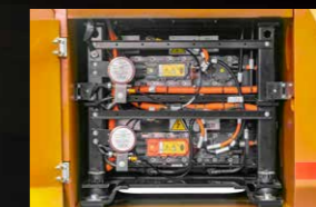
Battery and motor radiator
